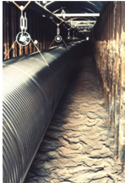
Figure 2 - The GEO600 vacuum pipe; 600 m long, 0.6 m diameter, 0.8 mm thick corrugated wall of 316L stainless steel.
